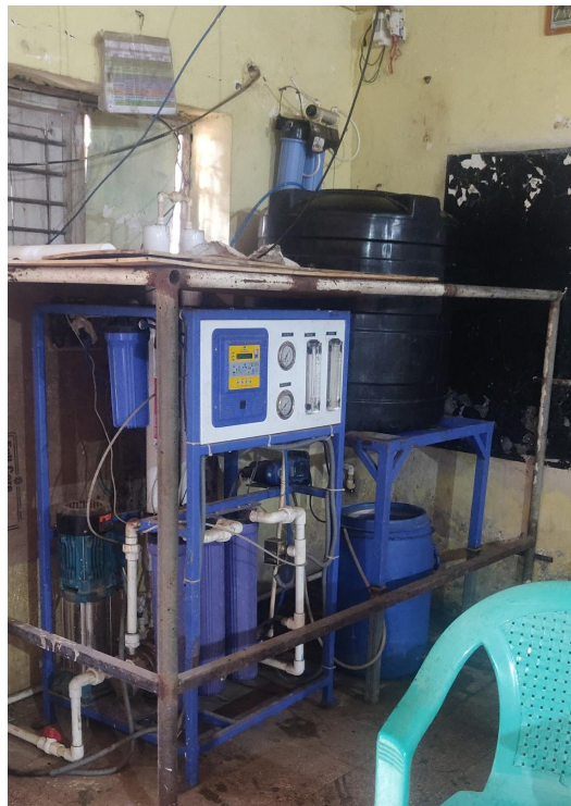
Figure 2.2.1: RO plant installed in a public school
